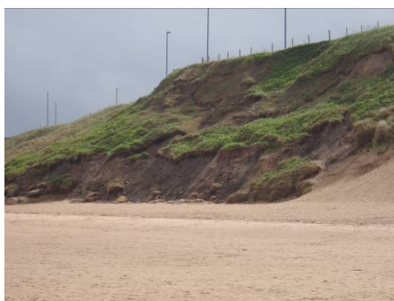
Profile NTDC06 – Measurable erosion of the dune toe
