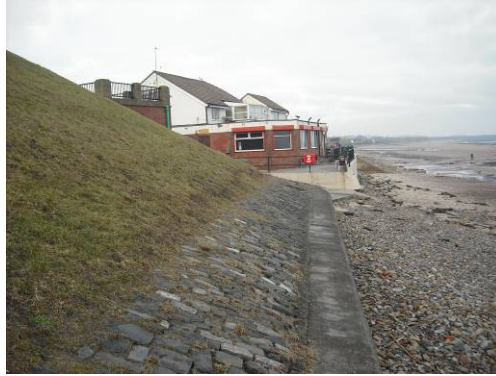
Profile NTDC04 – The surveyors noted an unstable slope, with small landslips and large cracks visible (not seen in photograph)
