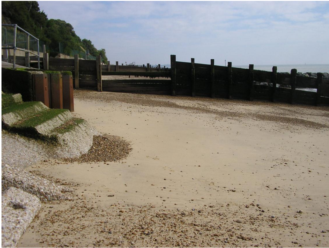
Photo 4: View of sea defences along the Felixstowe frontage in 2008 (location of EA survey transect S2A3). (Photo: Environment Agency)
