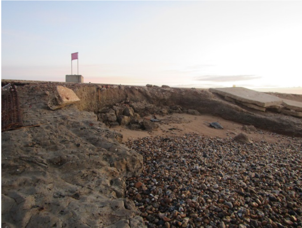
Figure 4- Erosion of the clay bund
