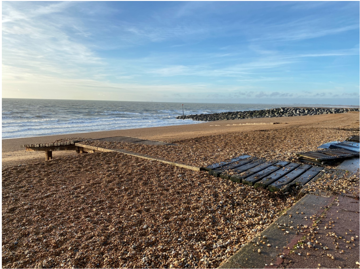
Figure 6 – Undermined ramp, and displaced boarding on promenade.
