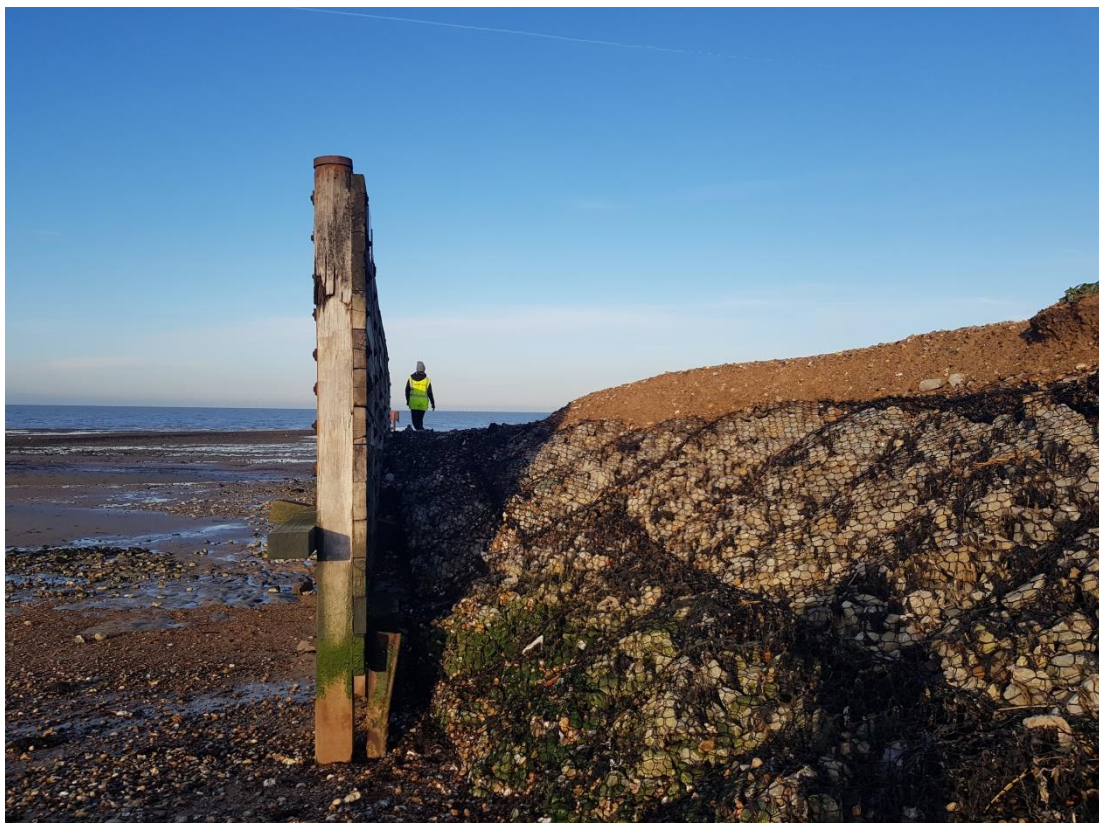
Figure 2.9 - Exposed mattress and outflanked timber groyne at the Tankerton and Swalecliffe survey unit boundary.
