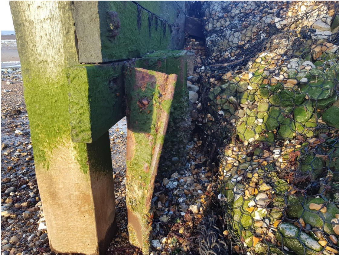
Figure 2.10 – Minor damage to sheet piling at boundary groyne.
